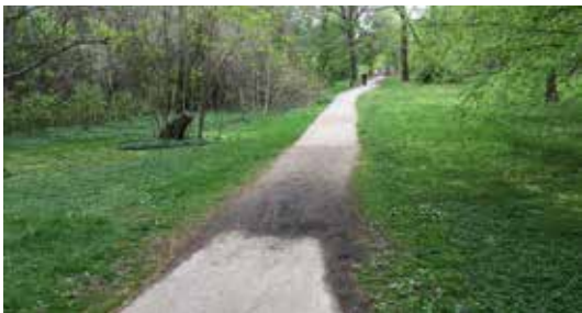
Area of poor drainage in Linkwood Park
