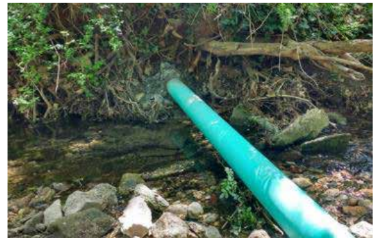
A Sewage-pipe leak received a short-term remedy
