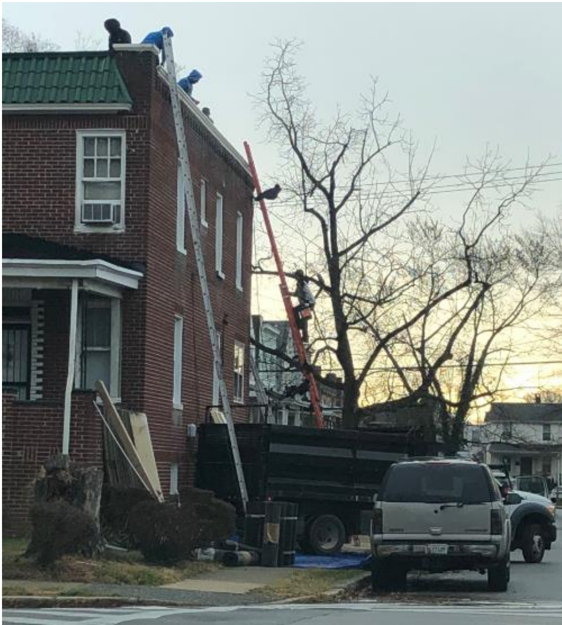
Homeowner Repairs near Arlington Elementary school in the INSPIRE footprint (1/4 mile around the school).
