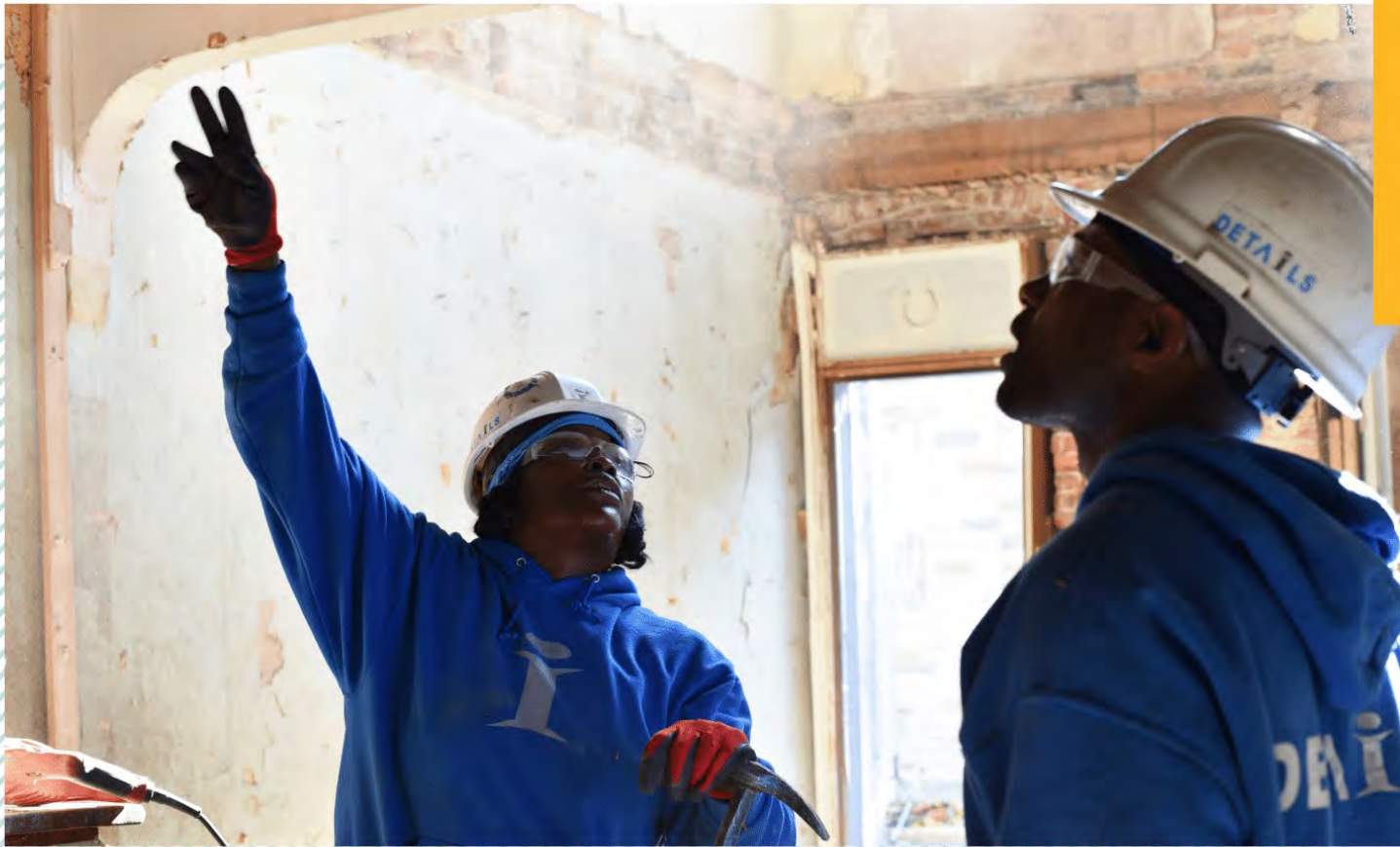
Employees with Details, a division of the Baltimore-based social enterprise company Humanim, work on deconstructing a home in the city.
