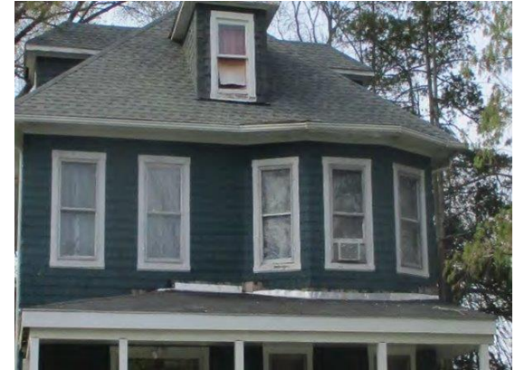
Before & After Window Replacement Done as part of the Lead Hazard Reduction Program
