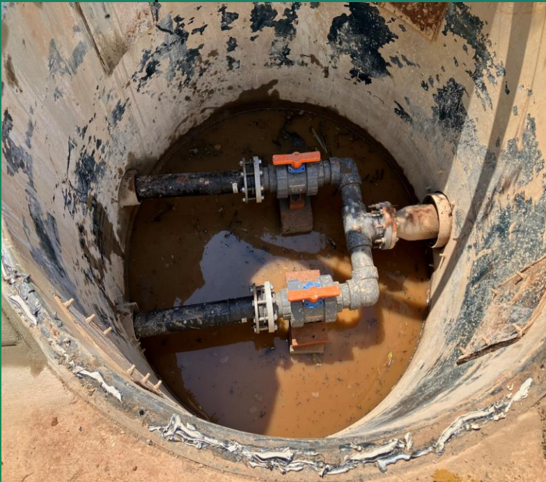
Intermediate Pump Station well with replaced connections.
