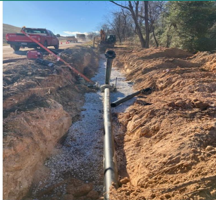
Leachate collection pipe install with Y clean out between Intermediate Pump Station and Leachate Lagoons
