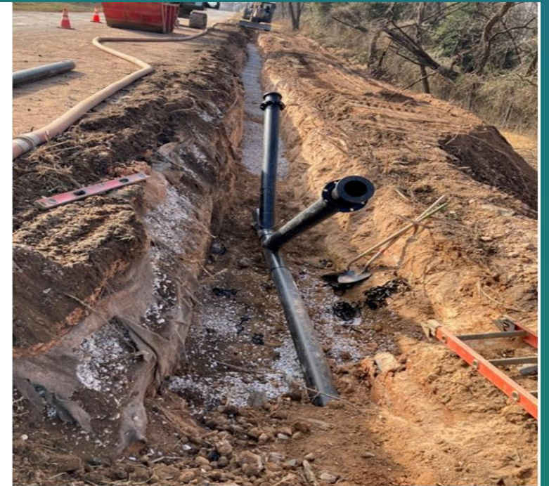
Leachate collection pipe Y clean out
